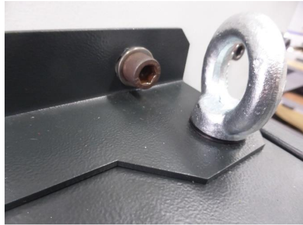
Photo No.22 / condition after testing. Jack ring (DIN580) and hexagon socket (M12)
